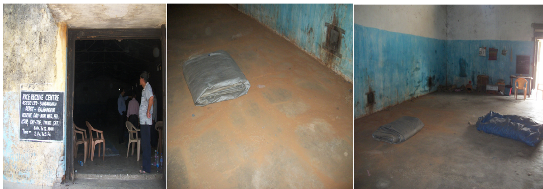
RRC at Sundargarh in wretched condition
