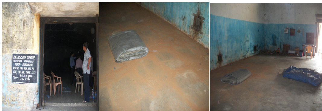
RRC at Sundargarh in wretched condition
