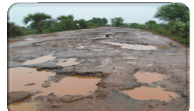
New Jagannath Sadak in deplorable condition - 13.60 km Picture No.2.4.4
