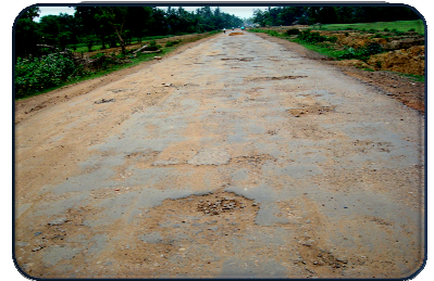
Cuttack Paradeep Road in deplorable condition at RD 18/300 km (Date:- May 2011) Picture No.2.4.1
