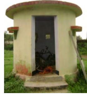
Unused sentry post at Jeypore Police Station used as cycle garage
