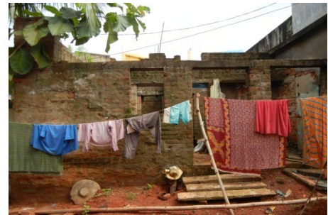
Delay in completion of dwelling units at Bharatpur slum noticed on 12 Sept. 2011
