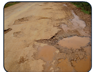
Cuttack Paradeep Road in deplorable condition at RD 16/00 km (Date:- May 2011) Picture No.2.4.2
