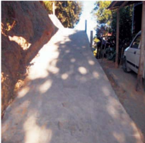
A photograph showing Construction of Stone Masonry steps with masonry pavement alongwith hand railing near Chawngkunga garage to Nunzami house, Luangmual (no hand railing provided)
