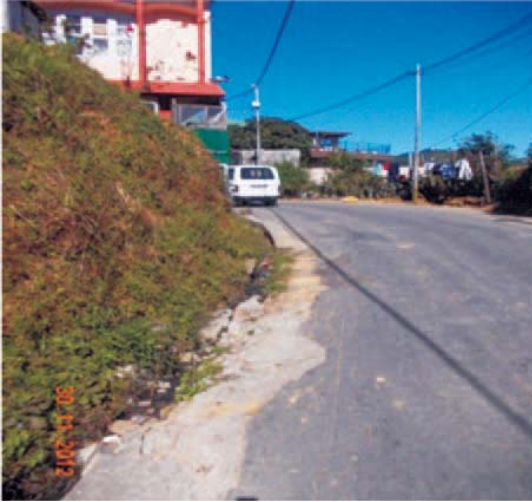
A photograph showing damaged section of the Construction of side drain near Pu Thangdailova (L)'s house to Pi Ruatsangi's house at Chaltlang.
