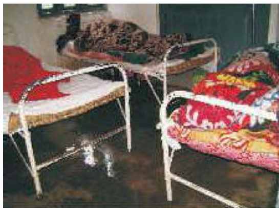
Stagnation of rain water in IPD of CHC, Janjehli (June 2010)
