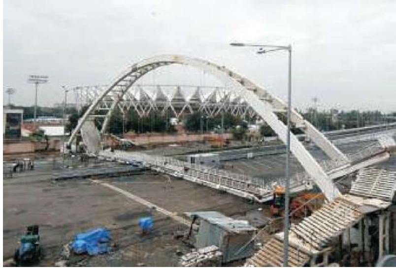
Collapsed FOB near JLN Stadium
