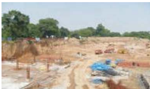
Picture of the construction site at Talkatora Indoor stadium indicating space available for construction activity.
