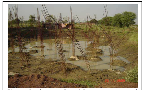
Picture showing water logged due to non progress of work and column steel has rusted at Mathpurena site - BSUP Raipur
