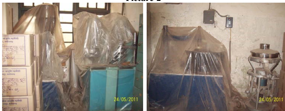
Idle machinery/equipment in Pharmacy
