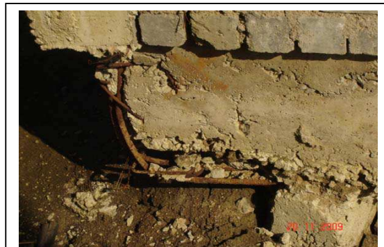
Picture showing eccentricity of Column at Mathpurena site – BSUP Raipur (The compressive strength of concrete work was found 111.15 kg/sqcm against the standard of 200 kg/sqcm.
