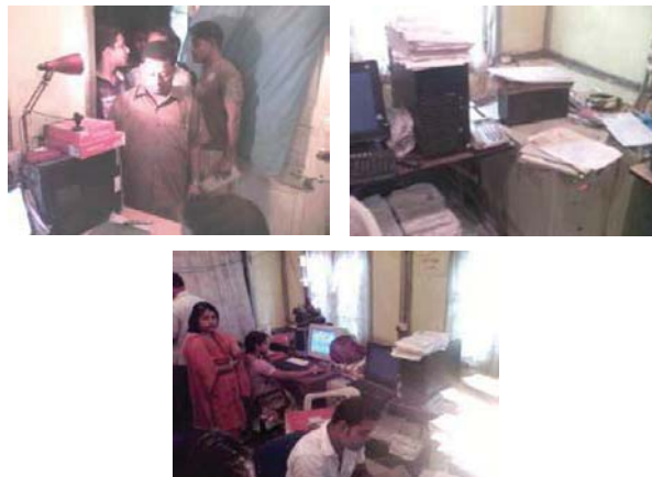
Pictures of server room of DTO, Nagaon depicting congestion, unrestricted entry and stocking of papers on the servers, UPS and batteries.
