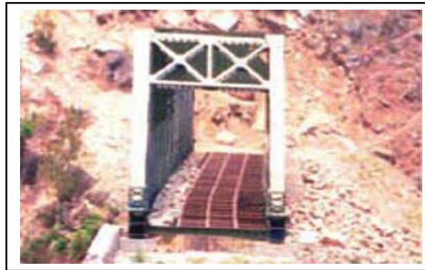
Incomplete and defective bridge over Tonse River
