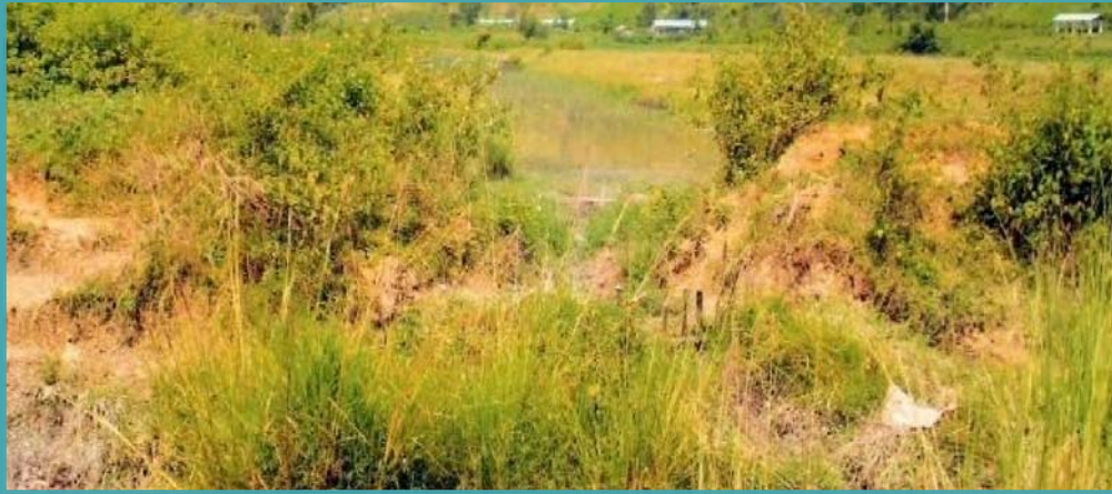
Thoubal Multipurpose Project – Manipur : Siltation, shrubs/weeds in Canal
