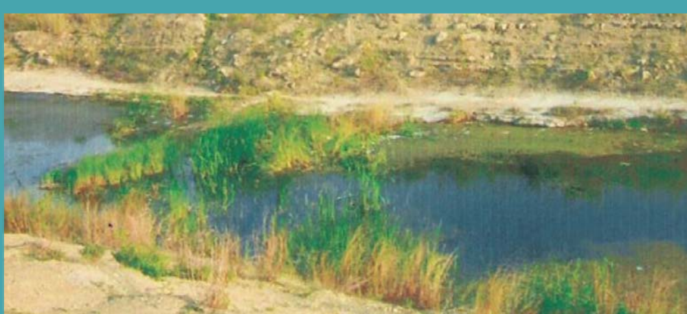
Right Bank Canal (RBC) of Rengali Irrigation Project – Orissa : Failure of slope and slippage of embankments at RD 31.55 to 34.24 km
