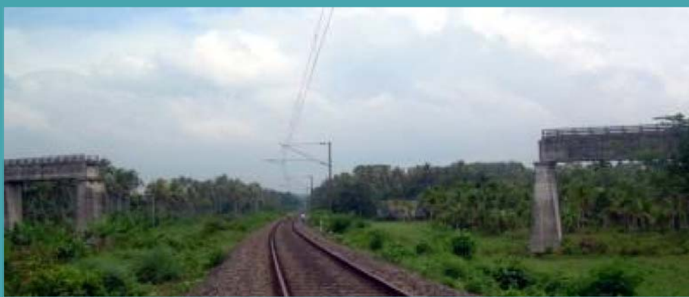
Muvattupuzha Irrigation Project– Kerala : Ezhuthonipadam Acquaduct - Bottleneck work in the Railway portion – Work yet to be arranged
