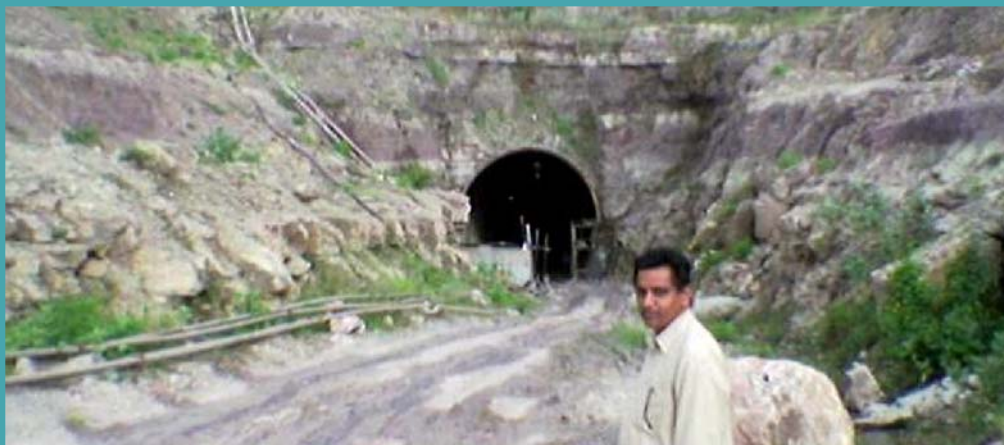
Bargi Diversion (Phase I) – Madhya Pradesh : Incomplete tunnel at Rd. km 33 to 35.42
