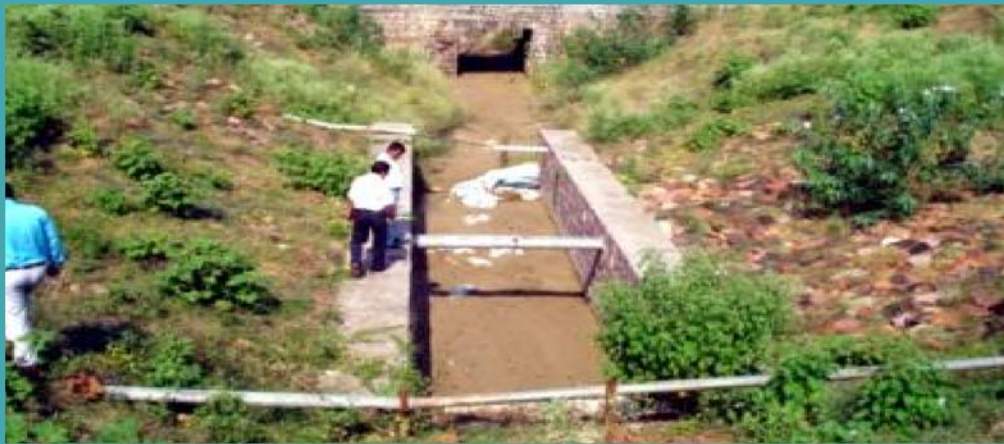
Rajghat Canal Project – Uttar Pradesh : Defective canal crossing at Km 0.750 of Bhailwara distributary below rail line and damaged canal due to back flow in the up stream of rail line
