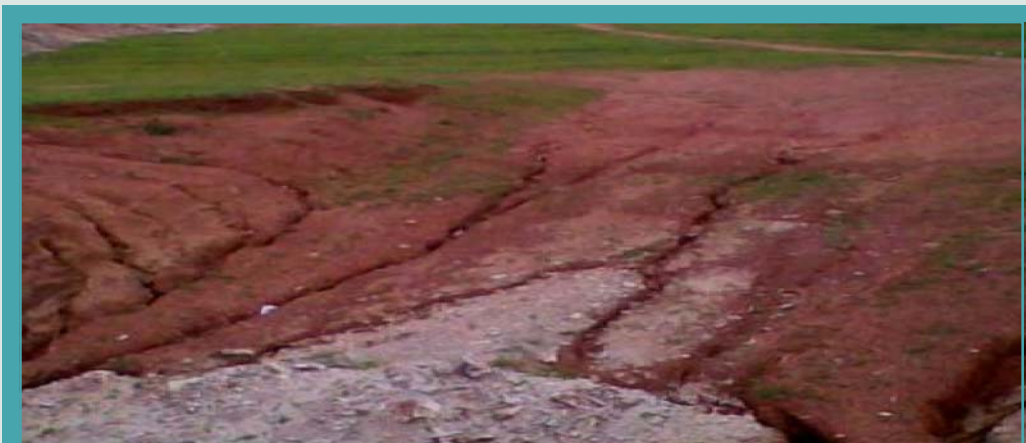
Patloi Irrigation Scheme - West Bengal : Work of proposed RCC Tunnel at chainage 551.20 in Purulia District held up due to land dispute.
