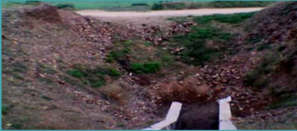
Bansagar Project (Unit-II –Canal) – Madhya Pradesh : Sihawal canal - Incomplete structure at Rd km 42
