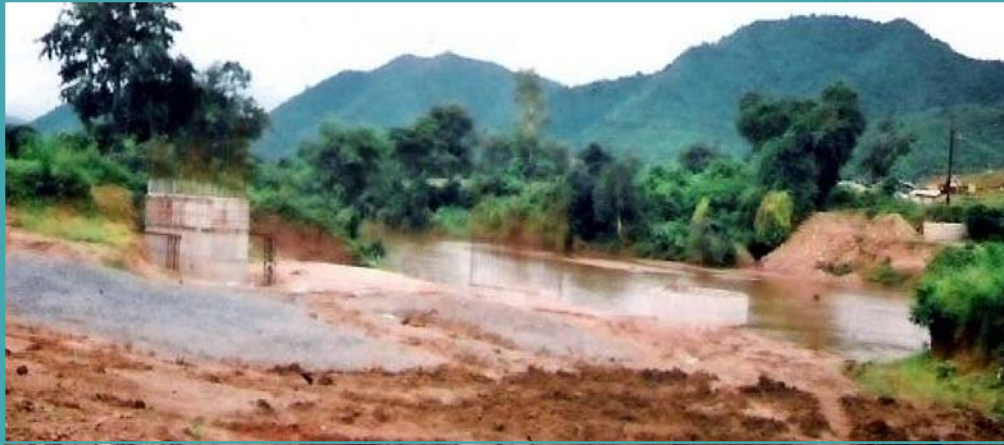
Upper Indravati Irrigation Project – Orissa : Syphon Aquaduct over river Sagada at RD 2820 M of RBMC remained incomplete due to non finalization of design
