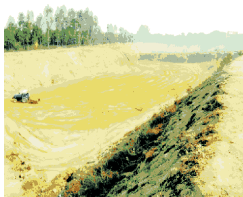
Development of site for Cell No.3 of CHWDF at Leather Cluster, Kanpur
