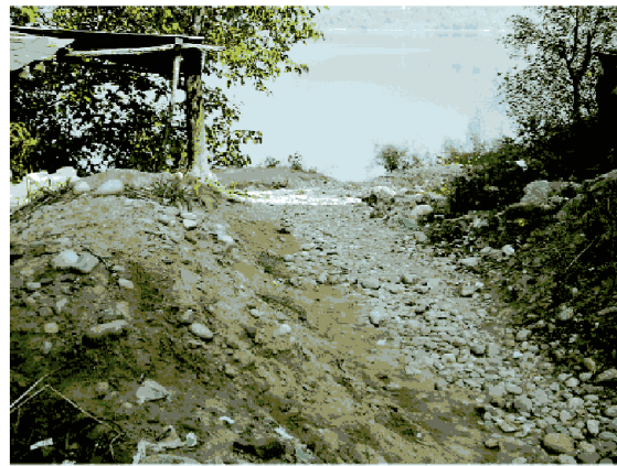
Jetty at Jeoripattan not constructed
