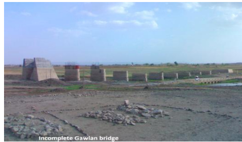
Incomplete Gawlan Bridge
