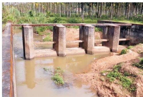
View of Vent Cross Bar
