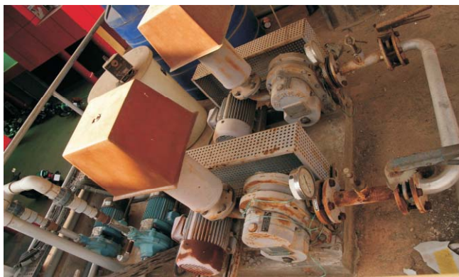
Parts of treatment plant got rusted
