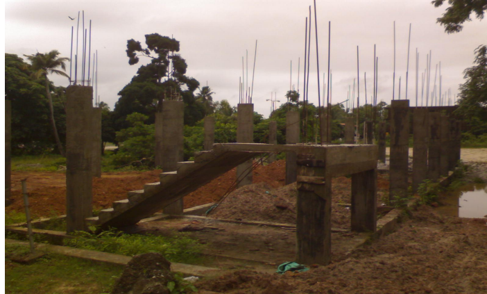
Incomplete building for outpatient in MCH, Alappuzha.
