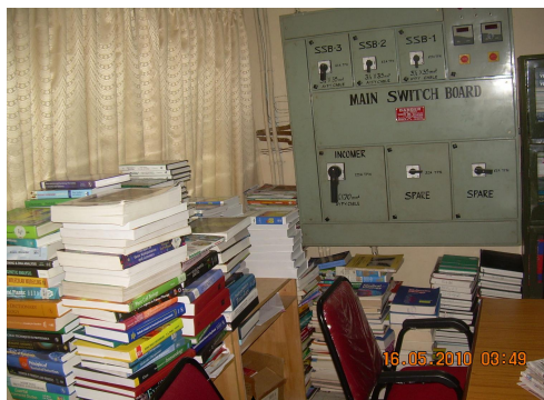
Library books stored near the main switch board
