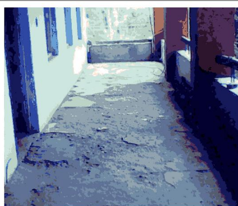
Damaged flooring of Police station Rajouri
