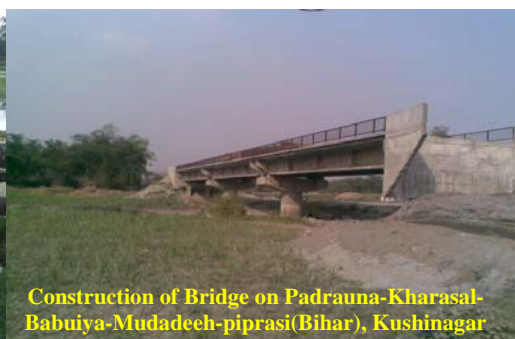
Construction of 4x5 m RCC bridge near Gram sabha Gaayghat and approach road
