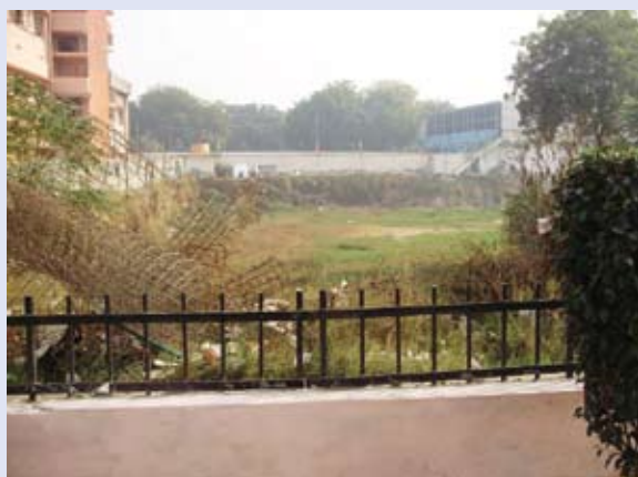
A view of excavations which endangered school property and lives of the students
