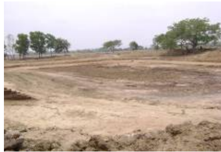
Bodhi tank at Latar of Ranapur block excavated using excavator and tractors
