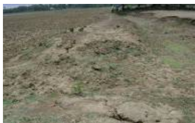
Road from Mandarkhanda to Pubasahi via Belapokhari (Gram Nandipur GP of Dasarathpur block) not fit for pedestrian traffic in summer months and inflated measurement with false muster rolls were noticed
