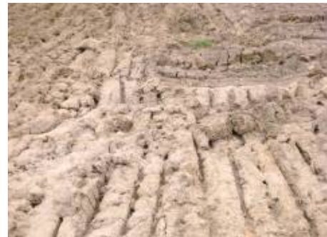
Digging marks of excavator in Bodhi tank at Latar of Ranapur block
