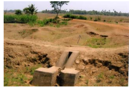
Damaged Manaour minor of Paika Rt distributary
