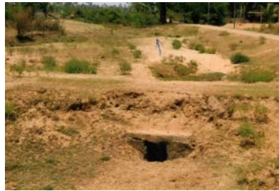
Silted up Olagada sub-minor of Mahanadi left distributary
