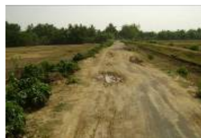
IC1 canal embankment road from Dhoda to Nandipur not providing all weather access after spending Rs 7.26 lakh by Dasarathpur block and overlapping execution by Irrigation Department
