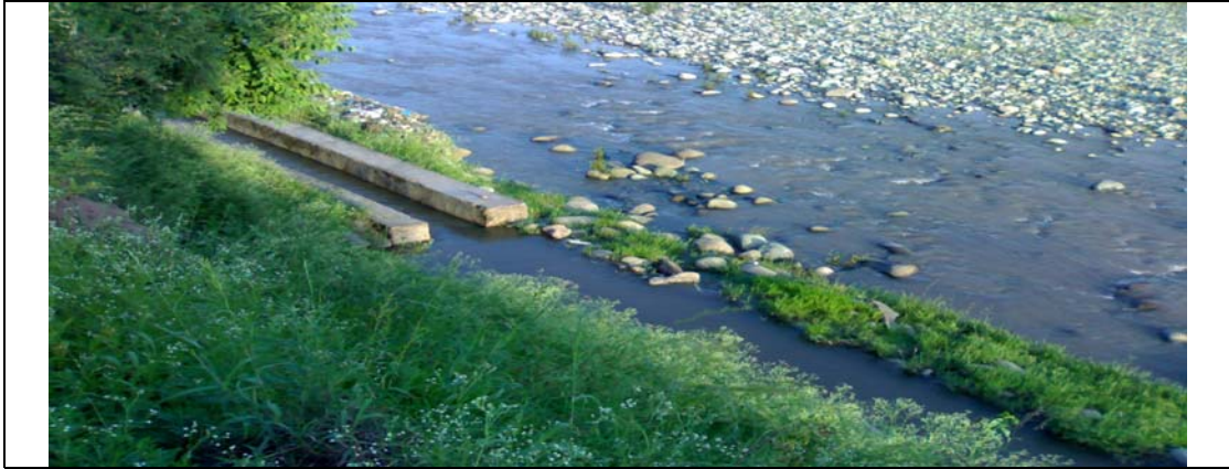
Poor intake head of Supply channel Narian.
