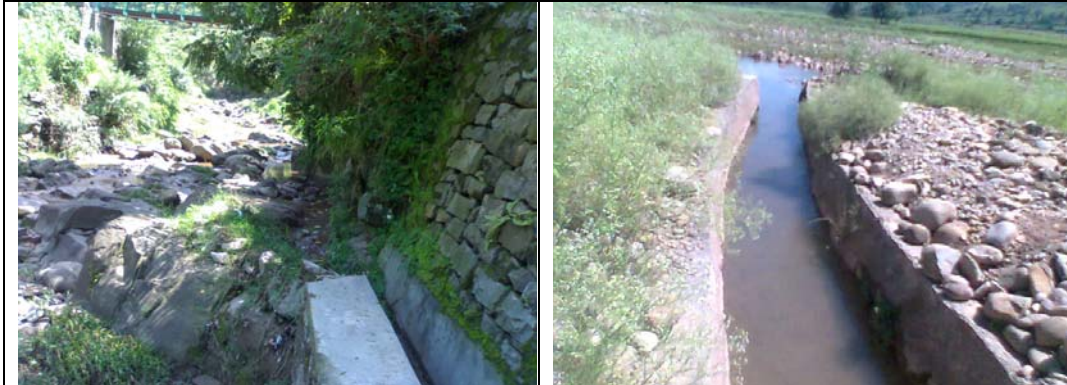
Regulatory System of Markas Khul not installed
