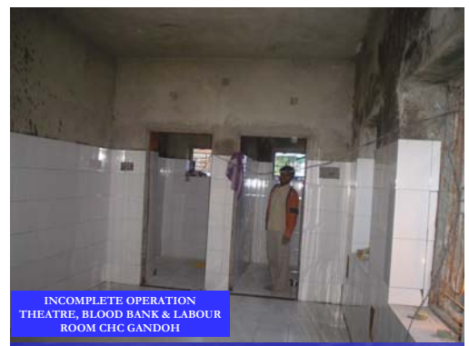
Under-construction Labour room, operation theatre and blood bank at CHC Gandoh, Doda. Equipment already received.
