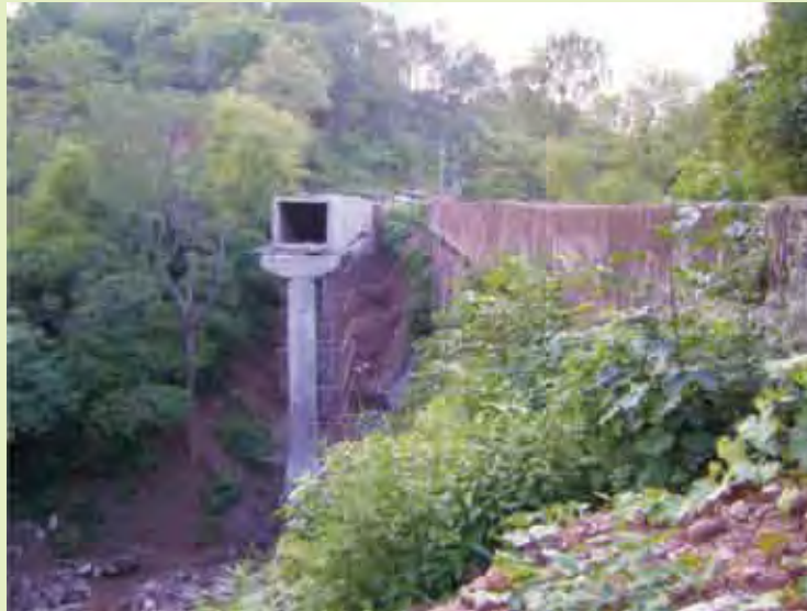
Aquaduct at kms 6.867 to 6.909 kms lying incomplete due to slow pace of work by the contractor
