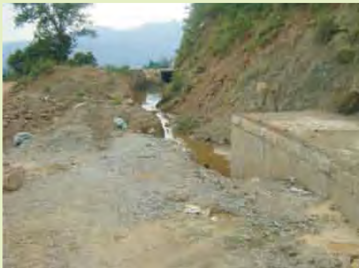
Portion of RCC Box where the work has not been done
