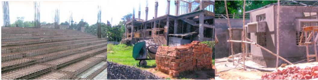
(Gallery, Front Elevation and Caretaker's Quarter of Joi Sing Doloi Auditorium Complex)
