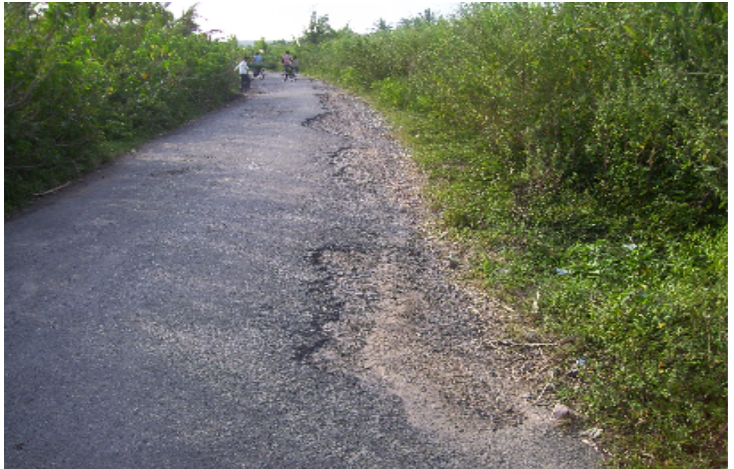
Status of road from BH Road to Tippalapura in Bhadravathi taluk
