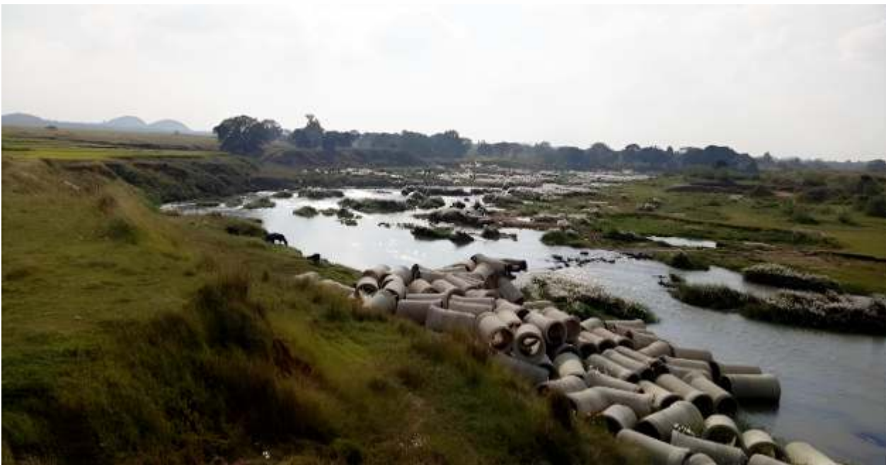
Incomplete main trunk line in the submerged areas of the river Jumar (20 October 2021)
