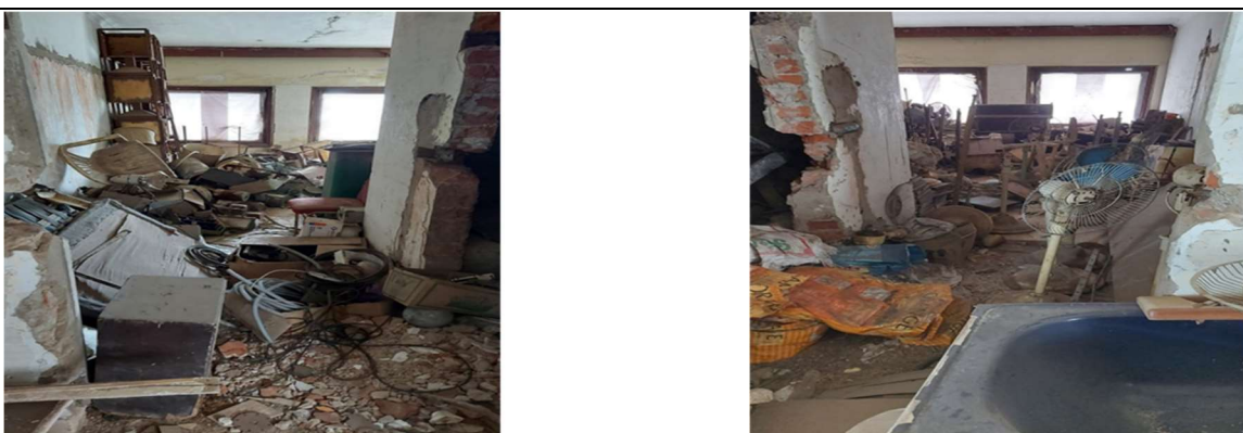
Picture 7.2: 28 rooms of Hotel Kalinga Ashok, Bhubaneswar remaining unserviceable
