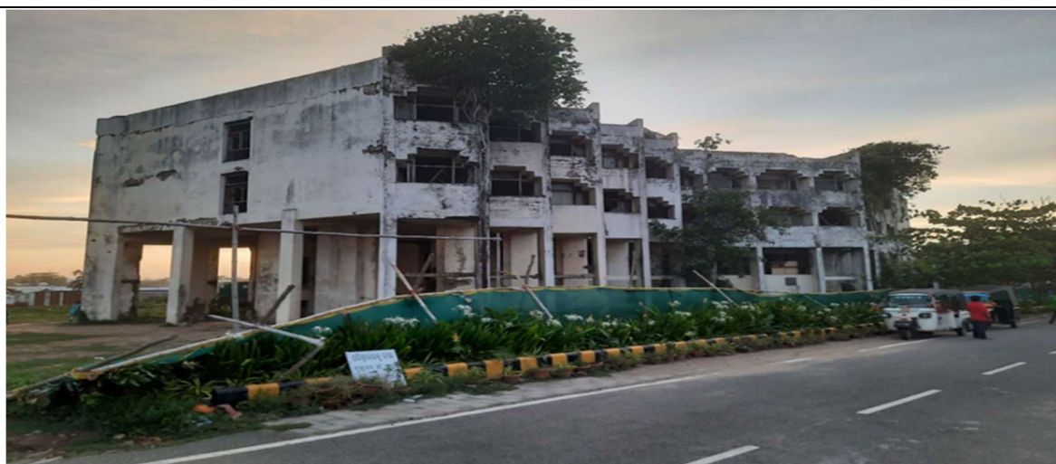
Picture 7.4: Dilapidated condition of Hotel Nilachal Ashok, Puri
