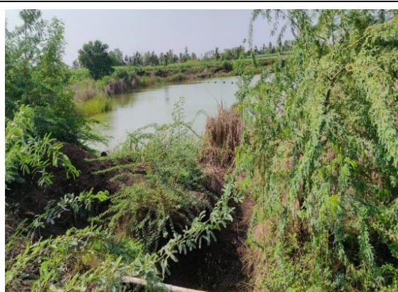
Image 1: Excavated Jack well (as per old design) and left unutilized due to shift in location of the Jack well
