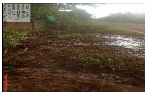
Picture No.13: Poorly maintained drainage at Honaga 1A, Belagavi
