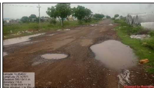
Picture No.14: Poorly maintained roads at Aliyabad 1A, Vijayapura
