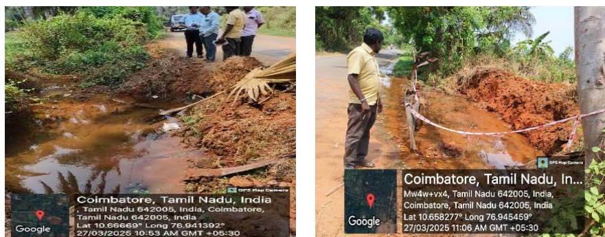
Exhibit 2.3: Water Stagnation due to leaks in pipelines
