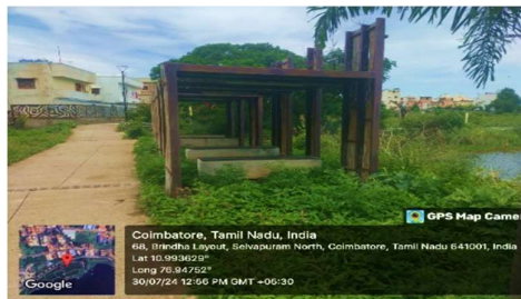
Exhibit 3.15: Poor maintenance of Selvachinthamani lake
