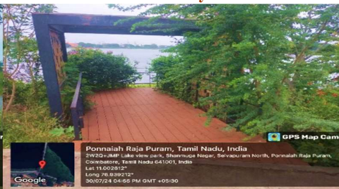
Exhibit 3.16: Poor maintenance of connecting bund of Selvampathi lake and Kumarasamy lake
