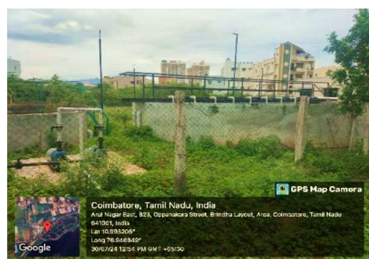
Exhibit 3.6: WWTP at Selvachinthamani lake not functional
