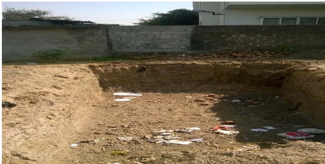
Picture 4: Open landfill pit in the residential area of Ward-B
