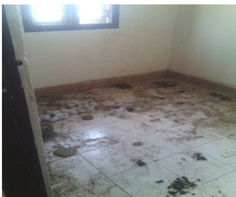
Picture 8 - Unallotted house at Rayanpalayam filled with debris and human waste
