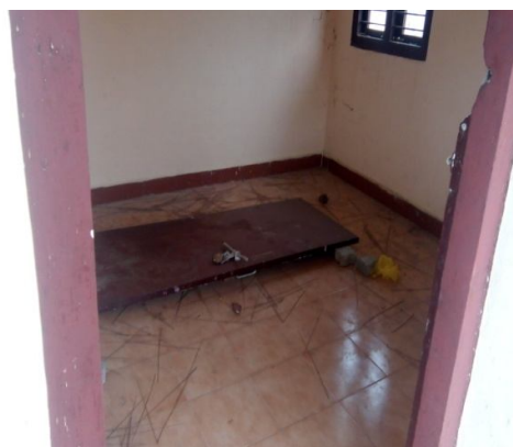
Picture 7 - A house at Manalipet where door was damaged by miscreants
