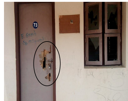
Picture 5 - A house at Ariyur where door was damaged and fuse box, fans and internal wirings were stolen
